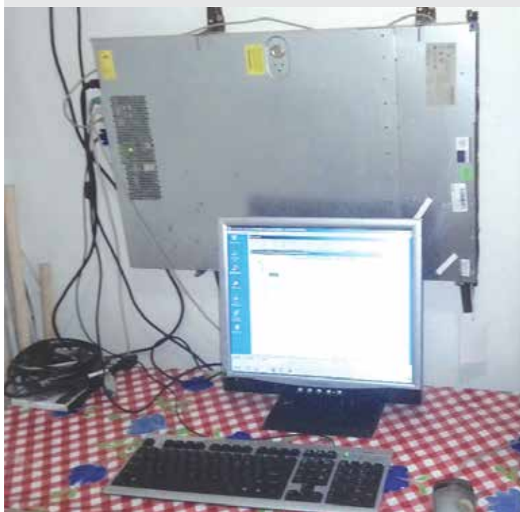
SAP server v serverovni / The SAP server in the server room
